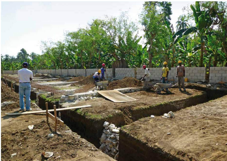
Reconstruction of the state school «Ecole Nationale de Dessources» in Léogâne, Haiti, has begun. The project is jointly funded by Liechtenstein and Switzerland.
